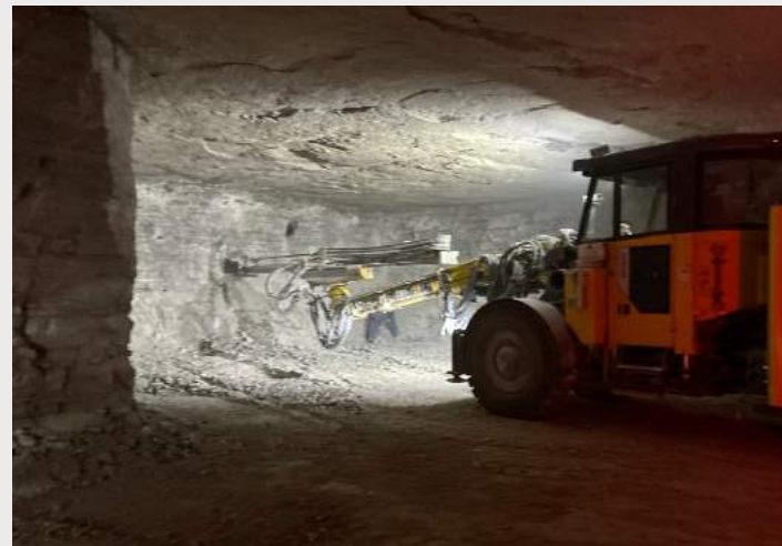
Drill operator Brandon Williams uses the drill rig to create blastholes in the rock for explosives placement.
