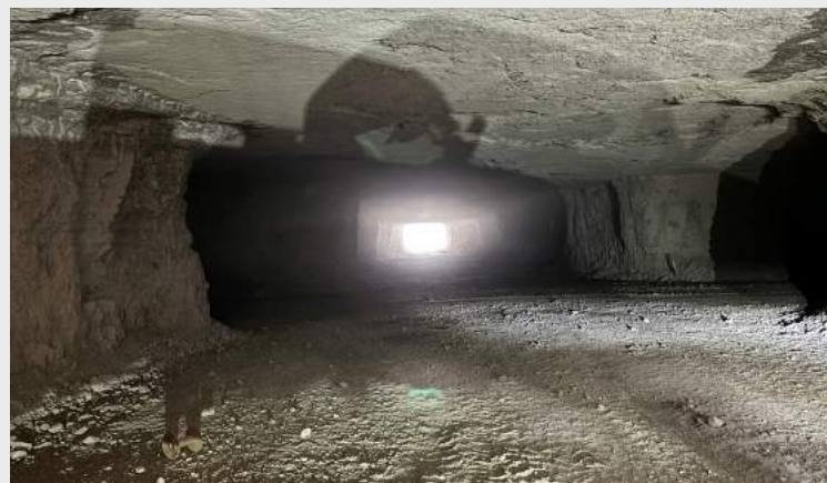
Pictured above is the portal from inside the mine. Crews are now working far enough back where they are unable to see the light of the entrance.
