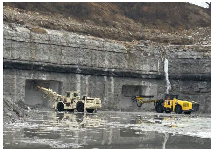
The scaler (left) and drill jumbo (right) work to create the two portals or entrances to the mine.
