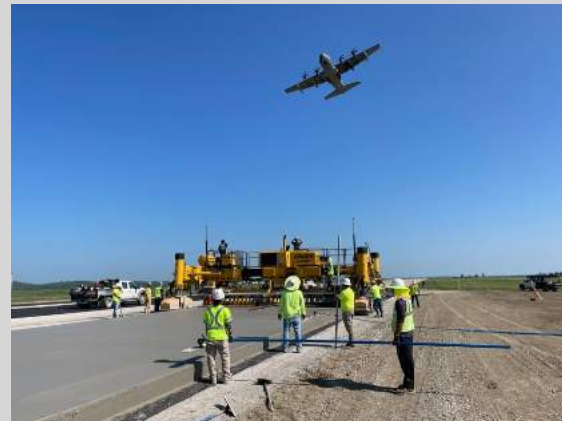
This season, crews were on high alert as planes took off and landed very close to the paving operations at Rosecrans Memorial Airport.
